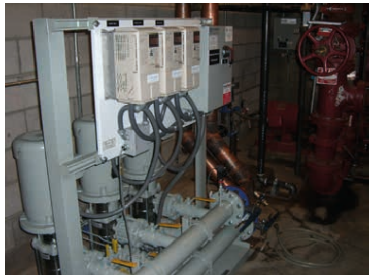
Examples of building booster station with three VFDs communicating serially for multiplexing without a PLC
