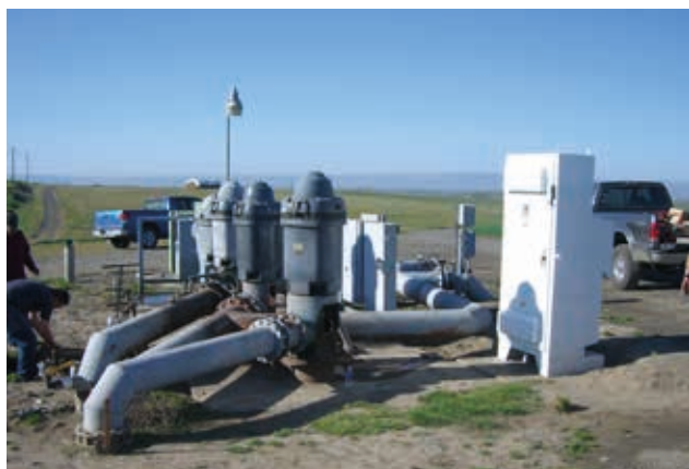
150 HP vertical turbines multiplexed with one running on VFD and three running across the line.
