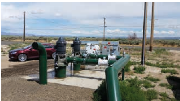
Two-pump system with one on the VFD and one running across the line controlled by the VFD
