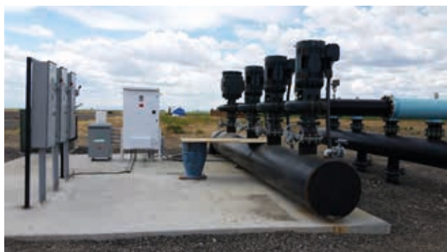
Four-pumps multiplexed on one VFD running one pump with the other three running across the line.
